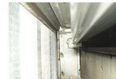
The UV light installation was not an easy one at Henry Mayo Newhall Memorial Hospital. There was no way to access the coil area.
