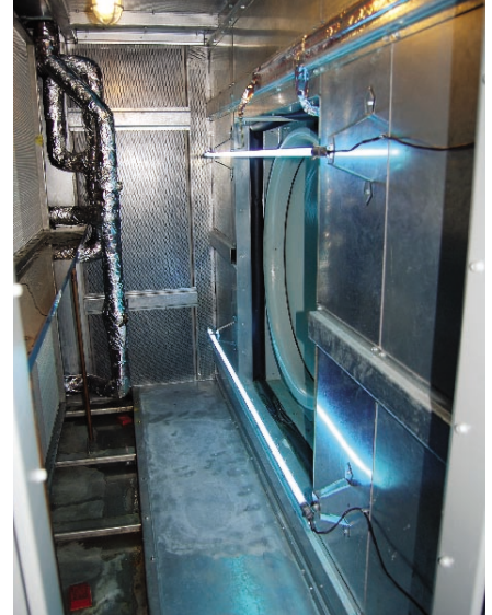
UVC lamps irradiating fan, plenum, and cooling coil, and all of the surfaces they reflect upon in a building owned by MGM in Century City, Calif.
